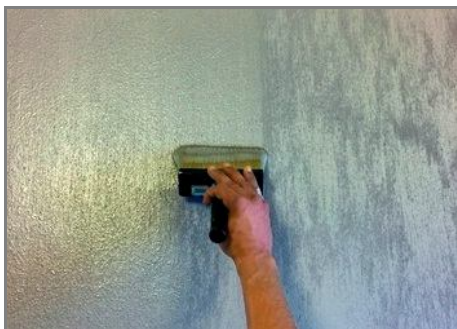
Step 5 - If desired, after a few hours, on a dry wall, apply a second coat to make the effect more full and homogeneous, keeping the vertical direction of the application and drawing FilidiSeta on the wall
