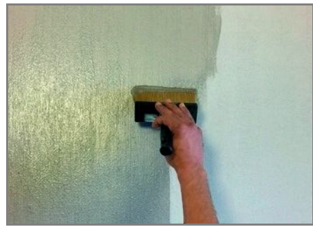
Step 4 - Distribute vertically the product on the wall, to maintain and draw the thready effect of FilidiSeta
